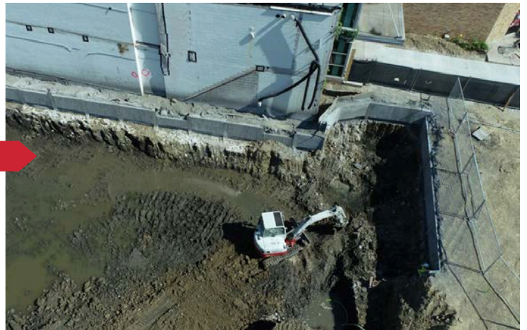
• 6/25/2024 The first lift of shotcrete at the soil retention wall. Each lift is 4' tall- three lifts total.
